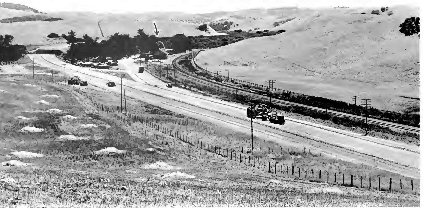
Realignment under construction at Pajaro River Crossing of U. S. 101. Arrow points to old one-way bridge on existing road
